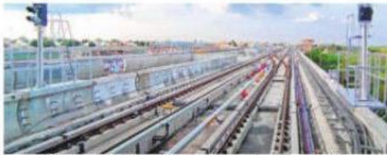
The Metro track at the station being built at Super Corridor. Signals are also being installed at stations
