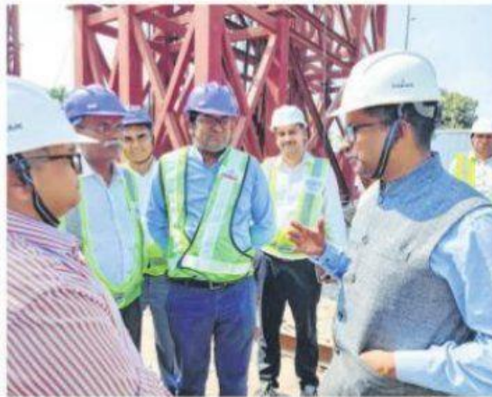
Madhya Pradesh Metro Rail Corporation Limited (MPMRCL) managing director Nikunj Kumar Srivastava inspects various construction sites of Indore Metro Rail Project in the city on Wednesday
