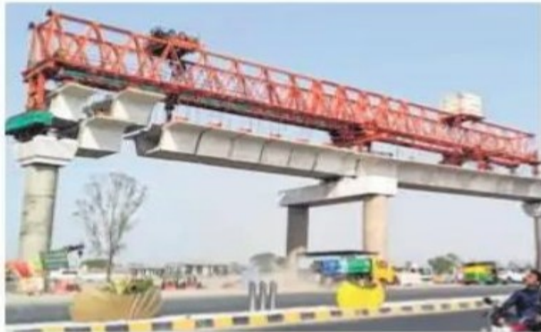
The work of Indore Metro is going on at the construction site on MR 10 where the slabs are being installed using a launcher. PIC BY - PINTU NAMDEV
