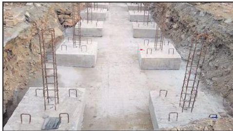
Metro Rail Corporation is developing platform for the first mock-up Metro coach at Shyamla Hills.
