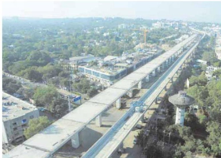
An arial view of the under-construction Bhopal Metro line near Rani Kamlapati Railway station in Bhopal on Tuesday. The deadline of the project is nearing fast, but almost 40 percent work is still pending. Pioneer photo
