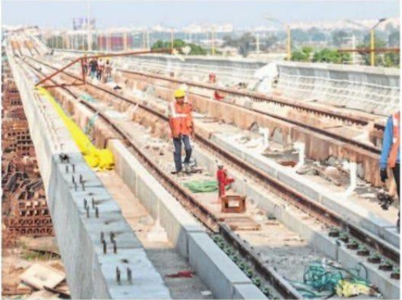
The laying of the second line of Metro Track at Super Corridor-3 started on Tuesday. PIC BY ANAND SHIVRE
