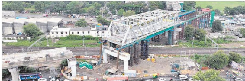
A bird's eye view of the railway over bridge (ROB) which was launched on Tuesday by MP Metro Rail Corporation.
