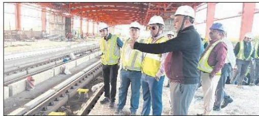
S Krishna Chaitanya, Managing Director of Madhya Pradesh Metro Rail Corporation, inspecting the ongoing works.
